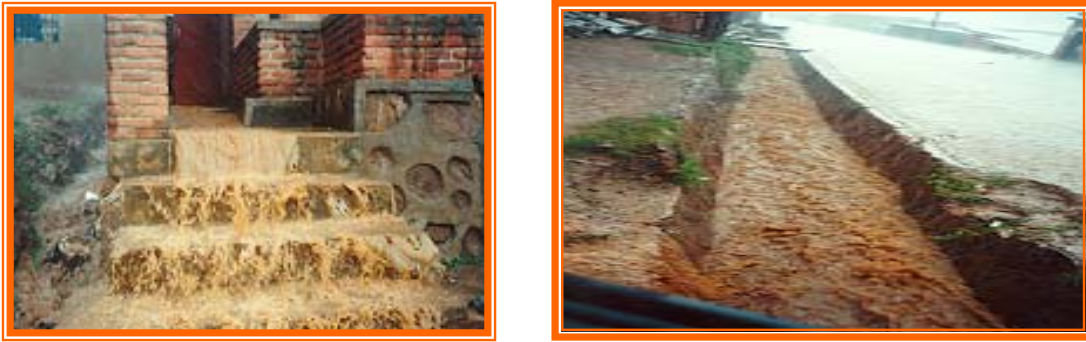
Photographs nos.6 and 7: After the rains, torrential water constitutes a danger as it destroys infrastructures in rural centres and cities
